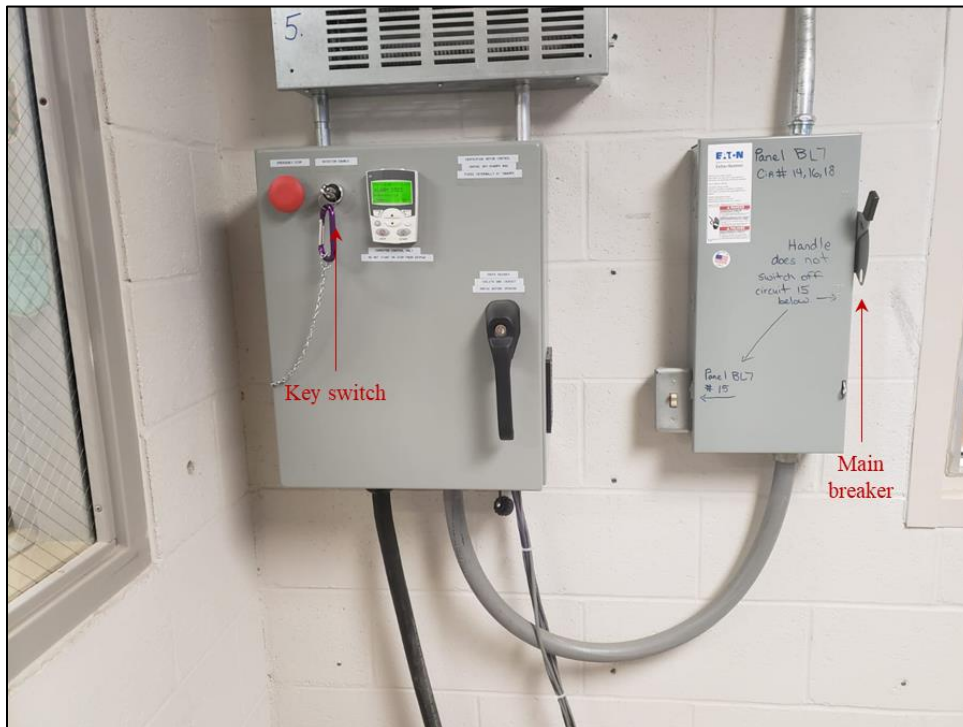
Figure A. 43 Main breaker and key switch to power centrifuge drive system.
