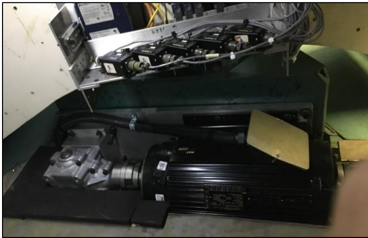
Figure A. 8 Electric drive system mounted in the centrifuge.
